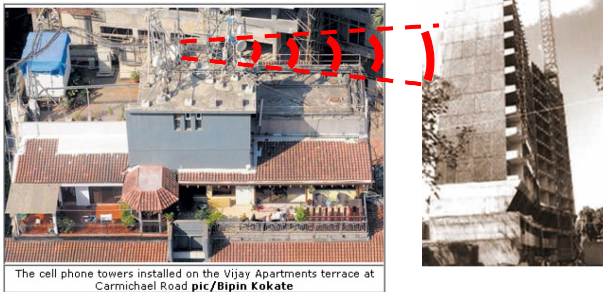
Fig. 2 – Cell phone towers installed at the roof top of a building in Mumbai
